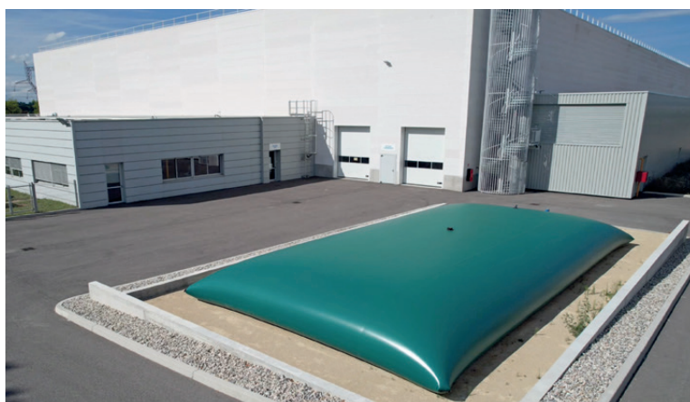
Fire protection tank
