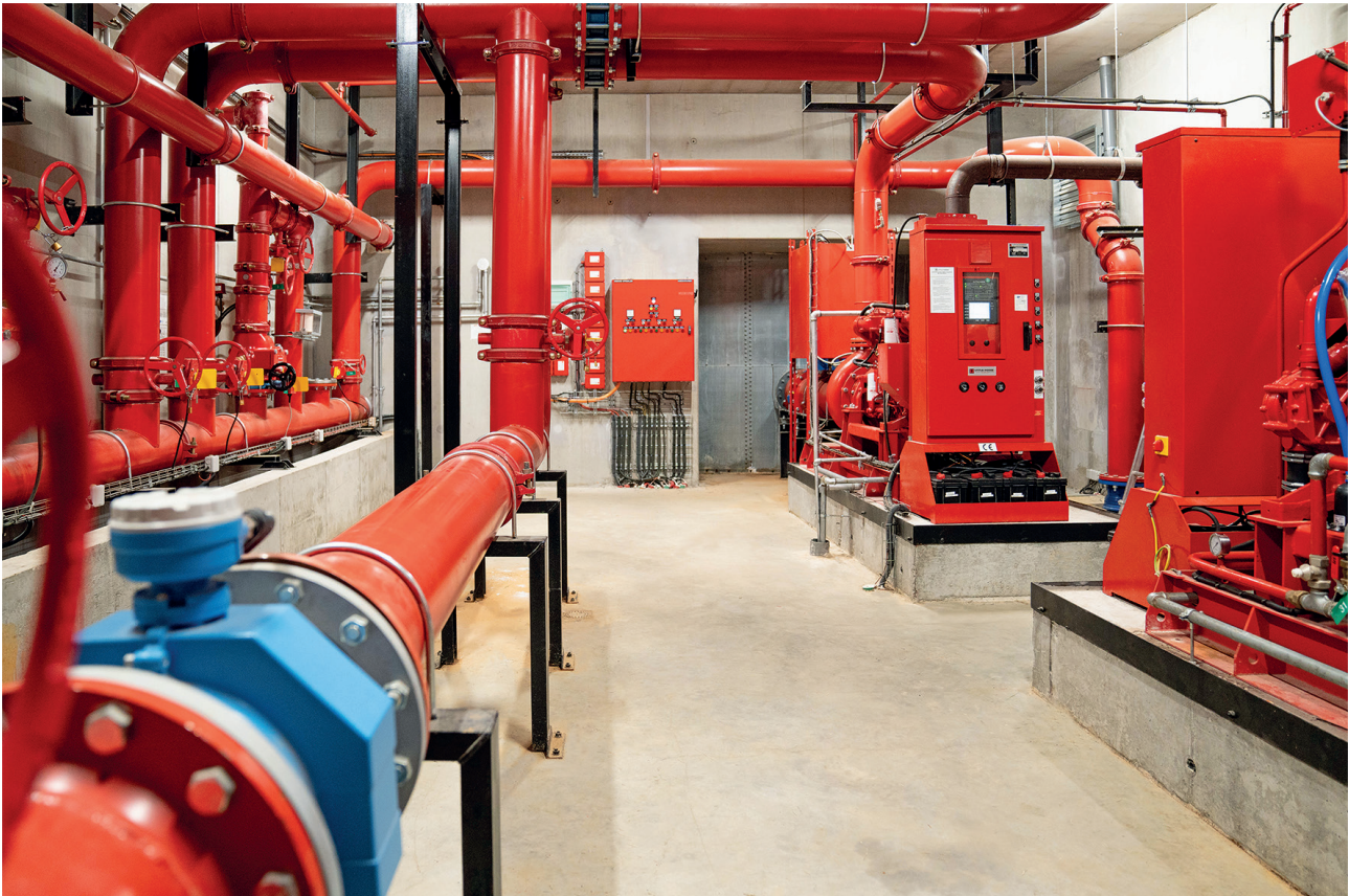
Sprinkler system at Odra
