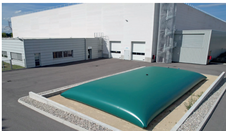
Fire protection tank
